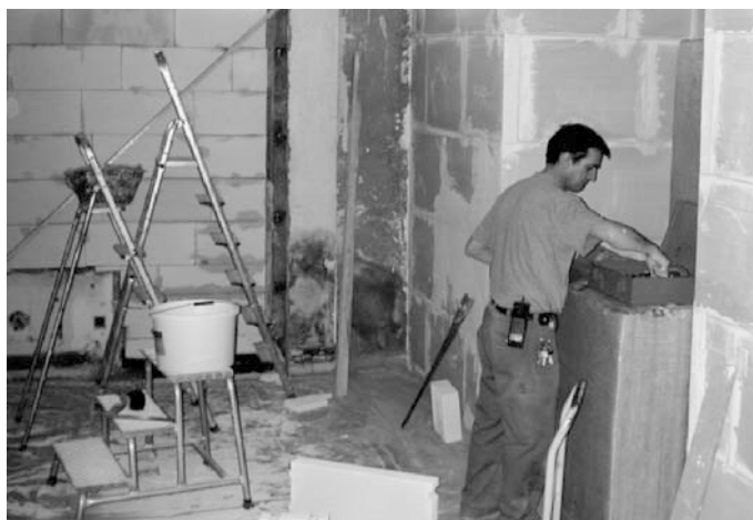
Paul Haas – our multitasking craftsman – was kept very busy with all the renovation work in 2003/2004. The picture shows him during the construction of the new server room (Photo N. Weiss).
